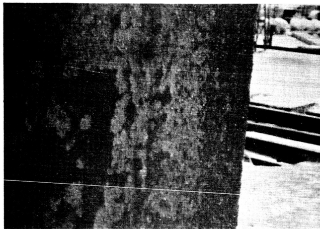
Fig. 16 Spalled Concrete on Southeast Corner of AGE Building, ETR Complex 40
